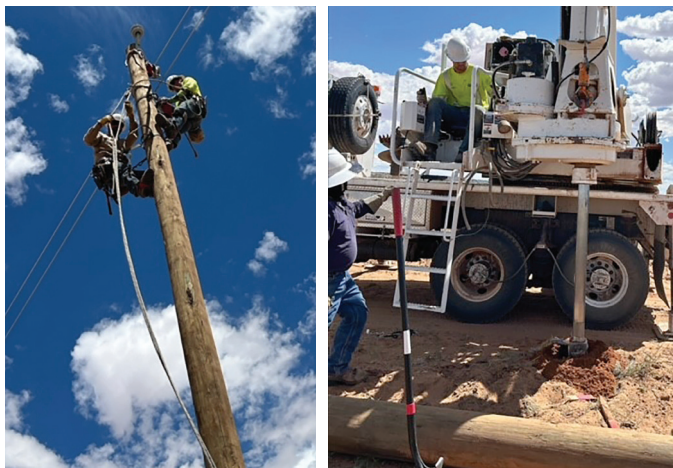
Left: While spending a week working on the Light Up Navajo Project, CWECC linemen Mack Yarbrough and Josh Wick climbed a lot of power poles. Right: Wick operates a pressure digger. Most of the pole holes required a pressure digger because of rock in the area.
