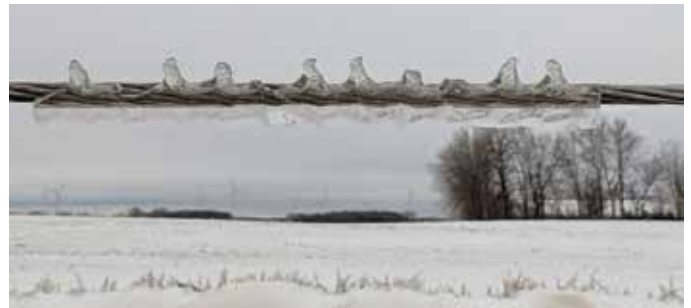
Below: Weight from ice-coated lines, combined with fierce winds, caused many of the poles to snap off at ground level.
